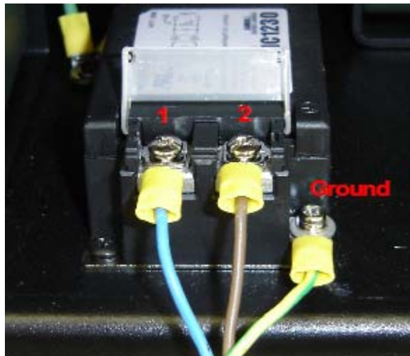
Figure 4 – AC power filter input connections
